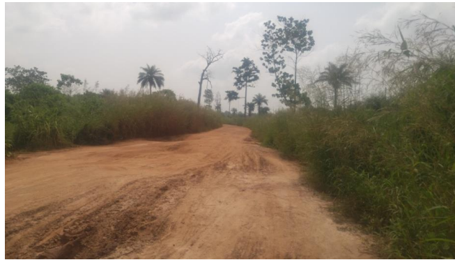
Figure 3.28: Poor Condition of a Secondary Road: Bo - Mattru Road
