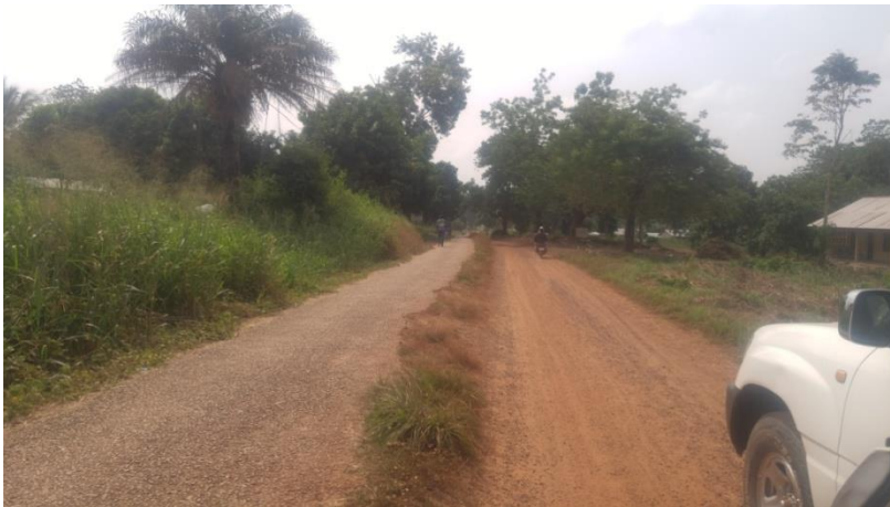
Figure 3.5: Evidence of Previous Surface Treatment Wearing Course on Road
