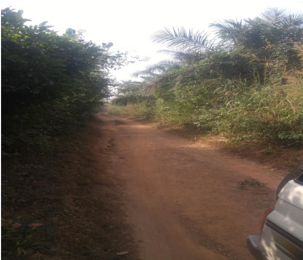
Figure 3.13: Virtually no gravel on surface; washed out.
